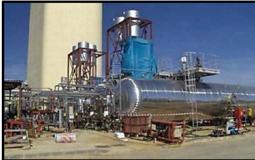
Figure 15: Energy Storage Tank at 10 MW Central Receiver ADS Plant in Seville, Spain (Medrano et al., 2010)
