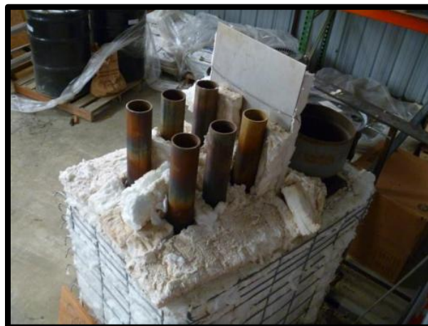
Figure 50: Insulated Salt Storage Tank
