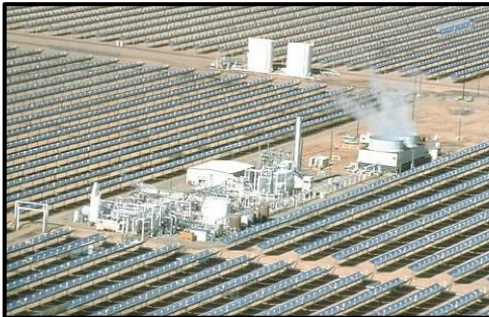
Figure 16: 10 MW SEGS I Power Plant and Trough Array in California (NREL, Parabolic Trough Power Plant System Technology, 2010)
