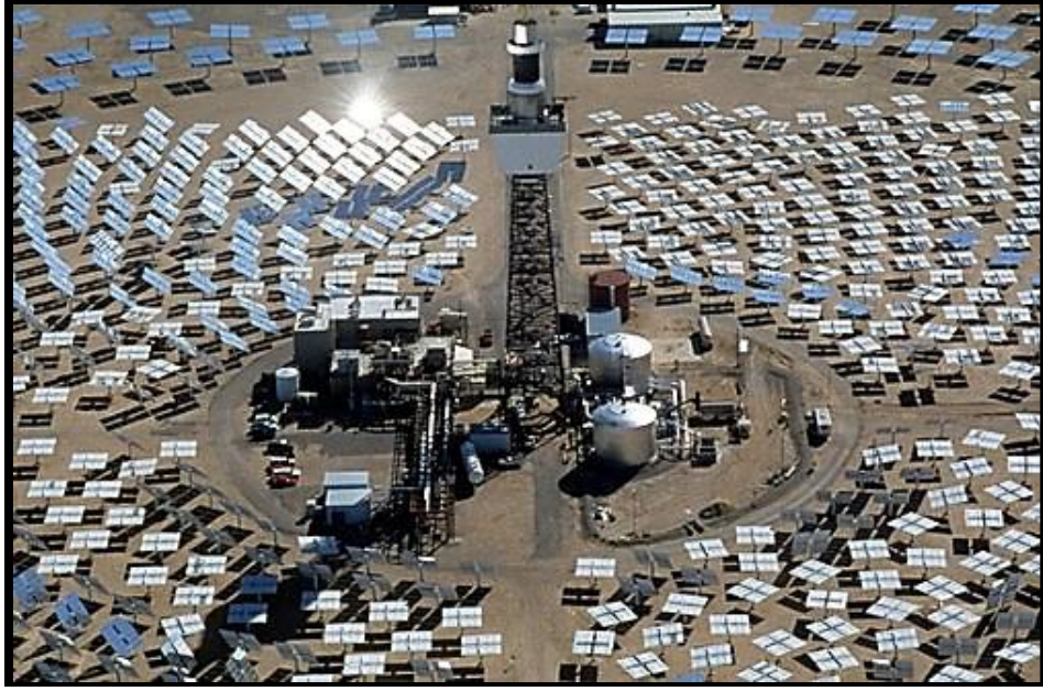
Figure 17: Central Receiver and Hot and Cold HTF Tanks at Solar Two in California (NASS, 2012)
